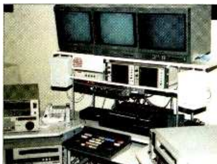
One of the two second-floor edit bays. Computer stands were modified to hold the necessary equipment.
